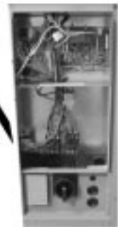
Control Box Access
